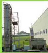
HMBR pilot plant location
